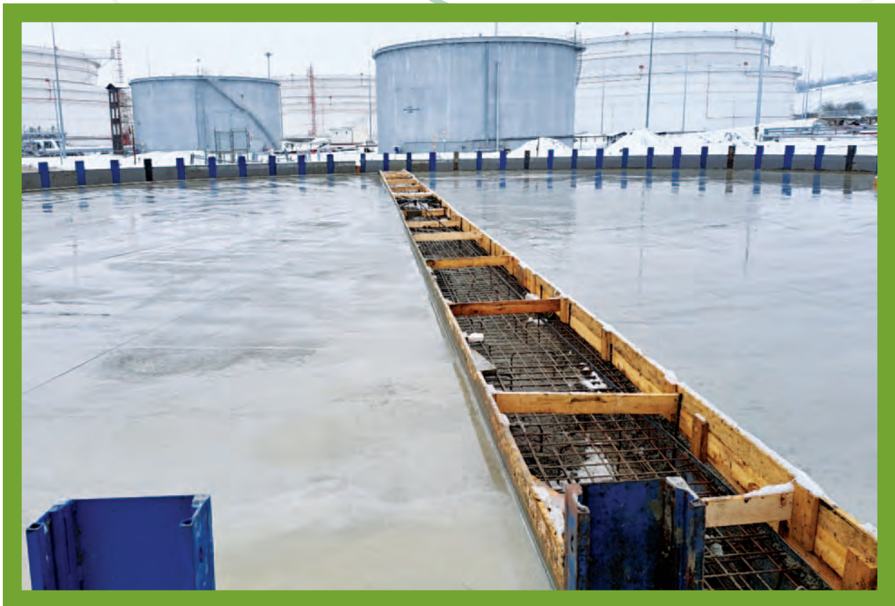
Photo: Work on the foundation of the new fire water tank; the original fire water and waste water tanks can be seen in the background.
