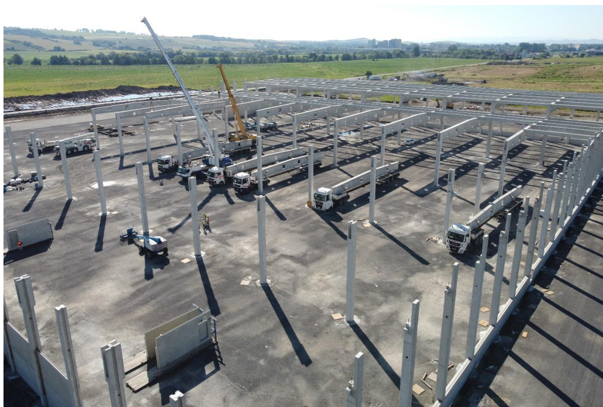
WINKELMANN installation, Rimavská Sobota
